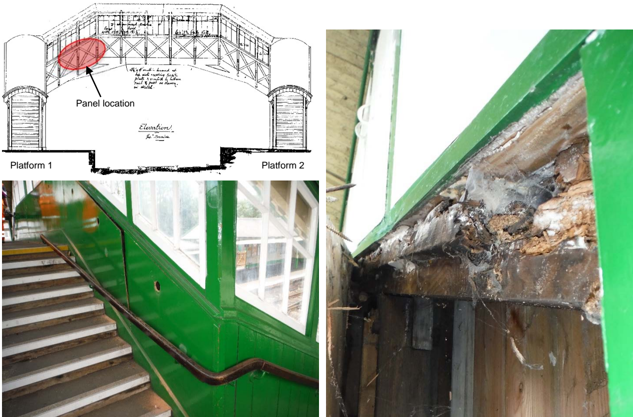
Figure 1: Location and rotten timber behind internal panel
