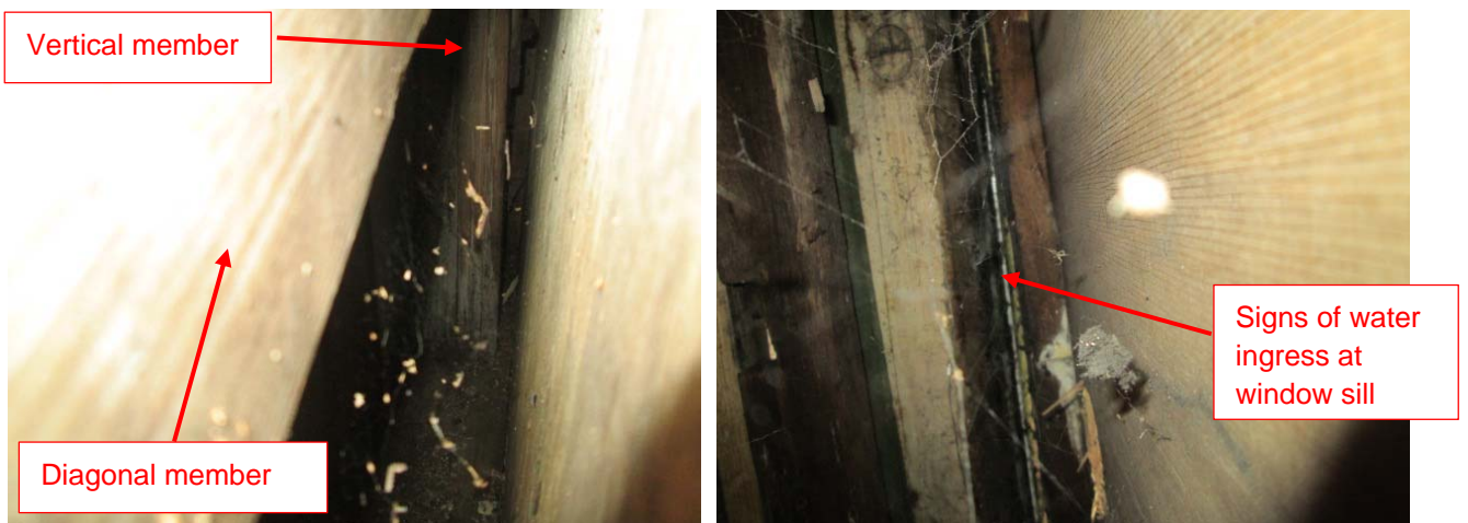
Figure 7: View towards Platform 1 and a view looking up to the window sill in Panel 5
